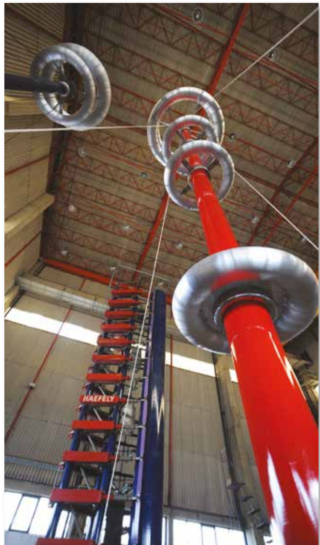
Lightning impulse generator voltage divider.
